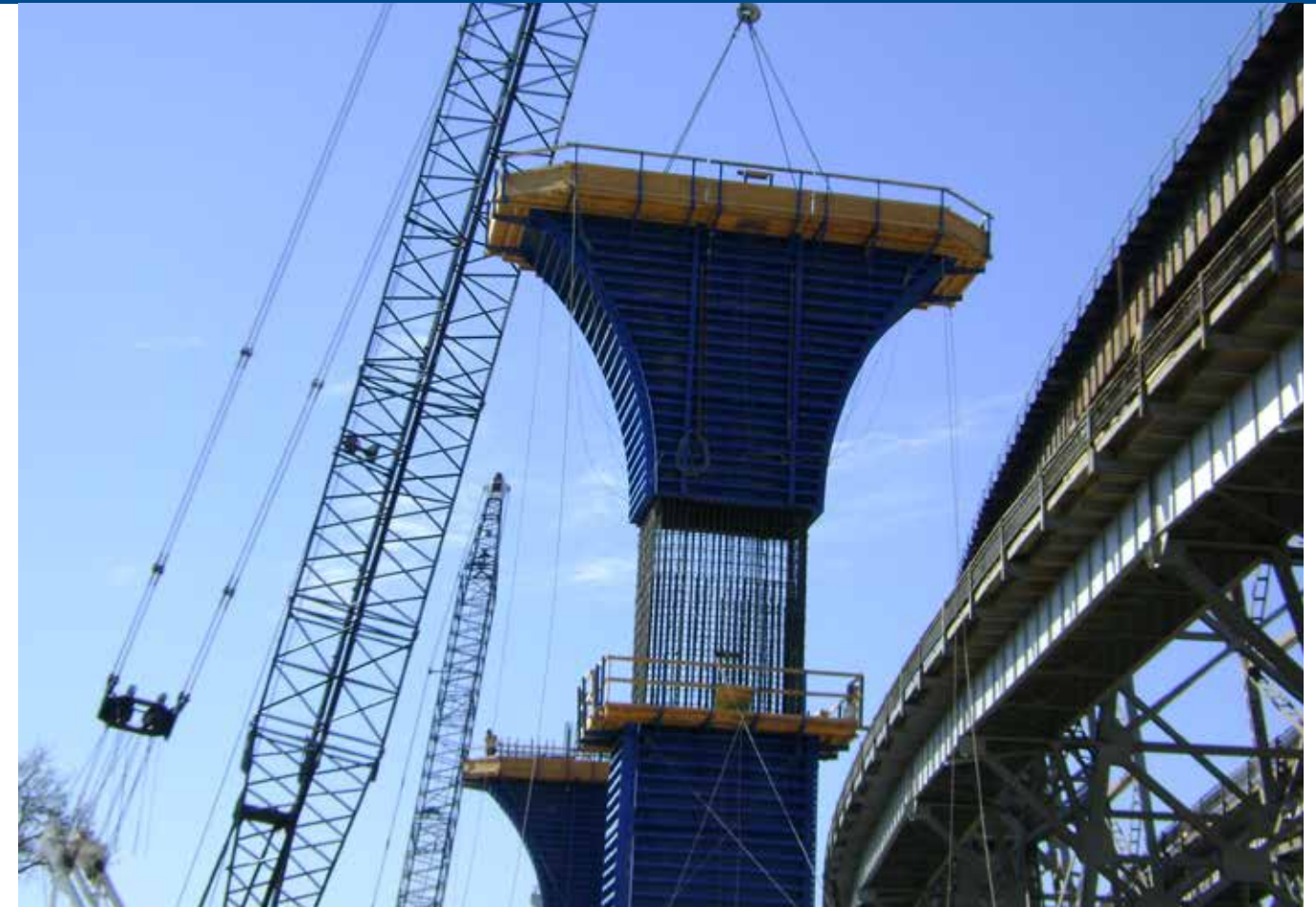
HP Long Bridge: Custom steel pier forms and flares on site in New Orleans, LA.
