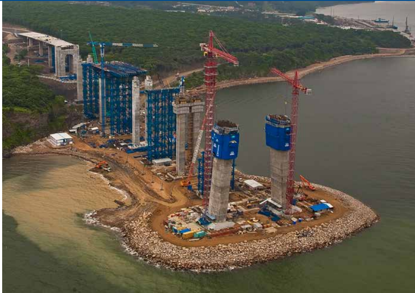
Russky Bridge: Construction of the bridge to Russky Island. The world's longest cable-stayed bridge, and the world's second highest pylons.
