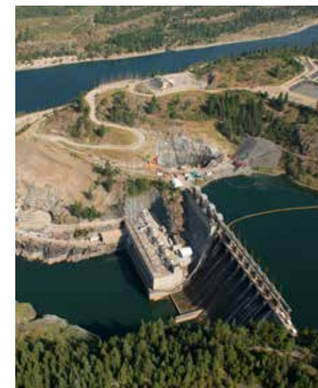
Construction of a new two-unit power plant commenced to increase the dam's generating capacity by an additional 335 megawatts in B.C. Canada.
