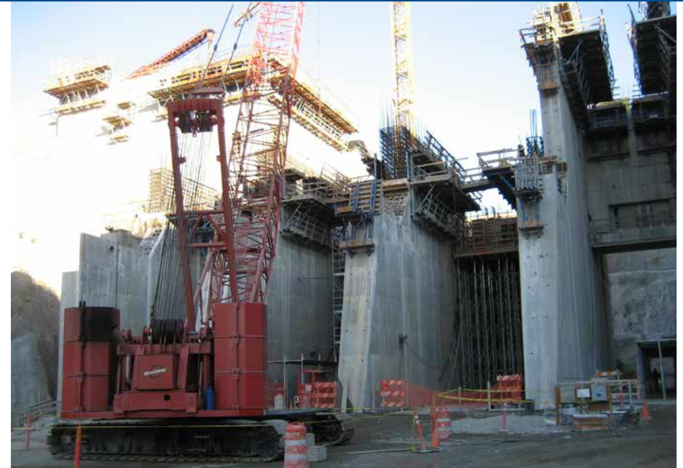
Folsom Dam: Climbing forms used in the construction of the massive concrete gravity dam on the American River of Northern California.
